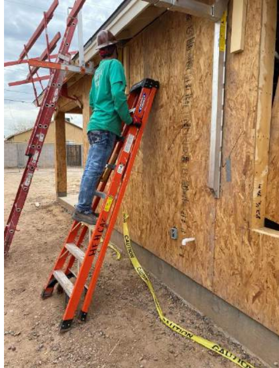
Never use an unopened A-frame ladder.
